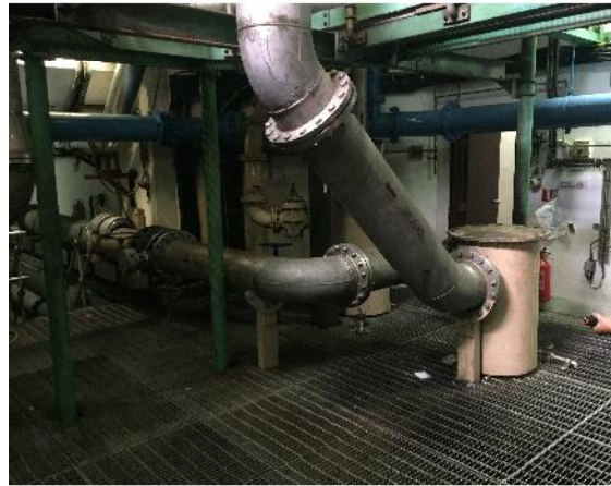
PHOTO 360: BIOGAS PIPES LOCATED IN THE BASEMENT OF METHANE COMPRESSOR HOUSE (DATE TAKEN: 22 MAY 2017)
