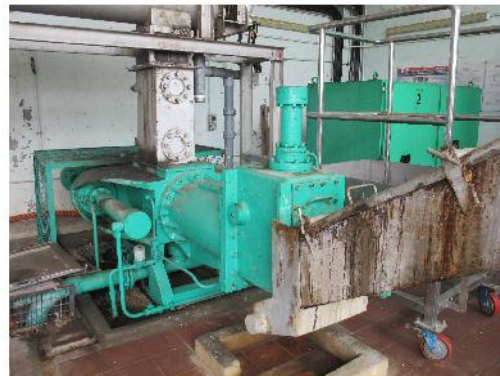
PHOTO 928: SCREENING PRESS NO. 2 IN SCREENING PRESS HOUSE (DATE TAKEN: 22 MAY 2017)
