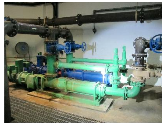
PHOTO 972: SLUDGE TRANSFER PUMPS LOCATED IN THE BASEMENT OF WATER HEATER HOUSE (DATE TAKEN: 22 MAY 2017)
