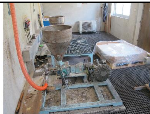
PHOTO 677: COAGULANT MIXERS AND COAGULANT STORED INSIDE CHEMICAL STORE ROOM (DATE TAKEN: 22 JULY 2016)
