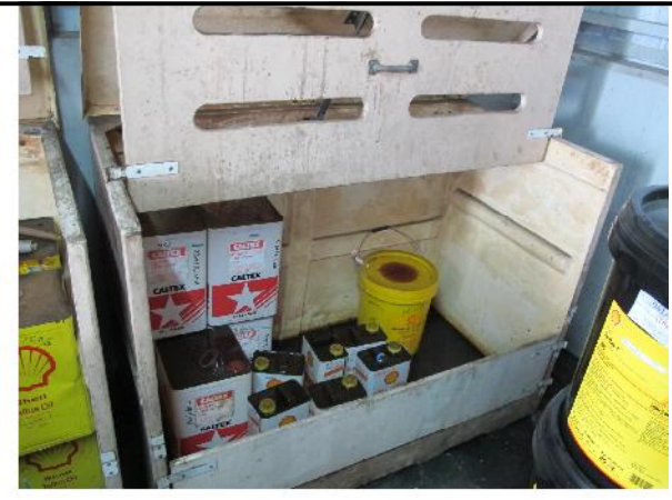
PHOTO 624: STORAGE OF LUBRICATION OIL IN CUPBOARD WITHIN LUBRICATION OIL STORAGE AREA (DATE TAKEN: 22 JULY 2016)
