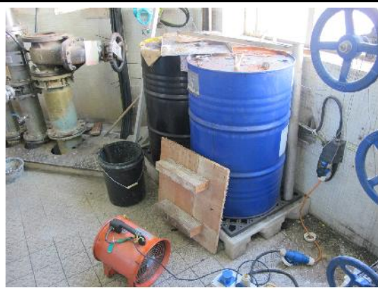
PHOTO 688: STORAGE OF OIL DRUMS ON PLASTIC PALLET ON THE GROUND FLOOR OF METHANE COMPRESSOR HOUSE (DATE TAKEN: 22 JULY 2016)
