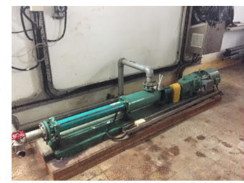
PHOTO 344: SLUDGE PUMP NO.1 IN THE BASEMENT OF SLUDGE DEWATERING HOUSE (DATE TAKEN: 22 MAY 2017)
