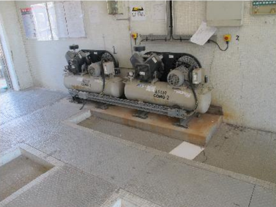
PHOTO 698: AIR COMPRESSORS IN WASH WATER PUMPING STATION (DATE TAKEN: 22 JULY 2016)
