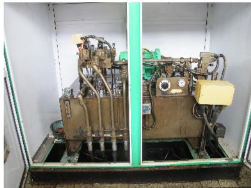
PHOTO 919: SCREENING PRESS CONTAINING HYDRAULIC OIL (DATE TAKEN: 22 MAY 2017)
