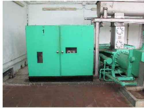
PHOTO 925: SCREENING PRESS NO. 1 IN SCREENING PRESS HOUSE (DATE TAKEN: 22 MAY 2017)
