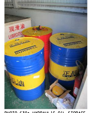
PHOTO 630: HYDRAULIC OIL STORAGE IN LUBRICATION OIL STORAGE AREA (DATE TAKEN: 22 JULY 2016)
