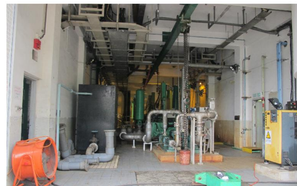
PHOTO 531: SLUDGE FEED PUMP ROOM ON THE GROUND FLOOR OF SLUDGE DEWATERING HOUSE (DATE TAKEN: 8 MARCH 2017)
