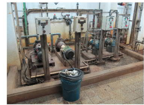
PHOTO 952: FERRIC CHLORIDE CIRCULATION AND DOSING PUMPS IN THE BASEMENT OF SLUDGE DEWATERING HOUSE (DATE TAKEN: 22 MAY 2017)
