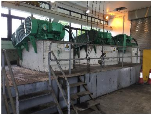
PHOTO 658: SCREW PUMPS IN SCREW PUMP PUMPING STATION (DATE TAKEN: 8 MARCH 2017)
