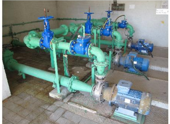
PHOTO 697: WASH WATER PUMPS IN WASH WATER PUMPING STATION (DATE TAKEN: 22 JULY 2016)
