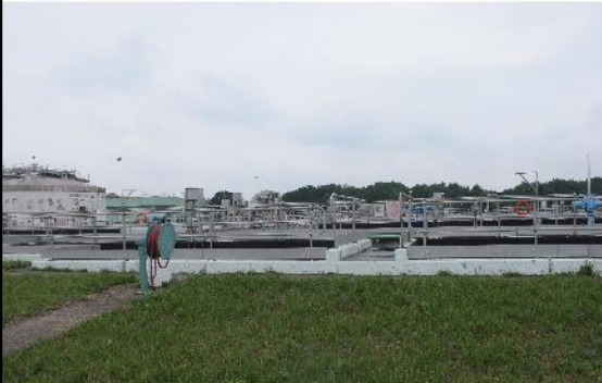
PHOTO 566: AERATION TANKS (DATE TAKEN: 8 MARCH 2017)
