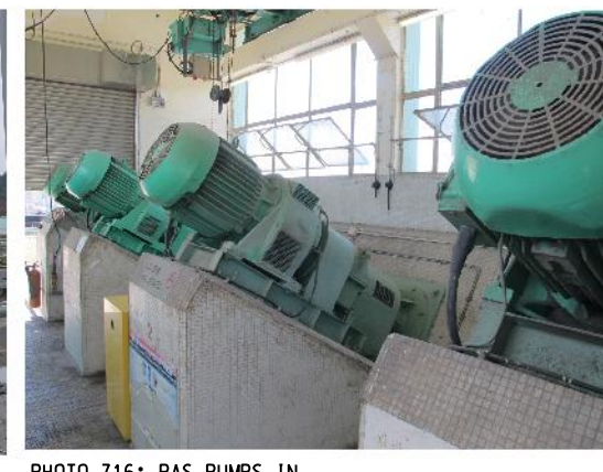
PHOTO 716: RAS PUMPS IN RAS SCREW PUMP PUMPING STATION (DATE TAKEN: 22 JULY 2016)
