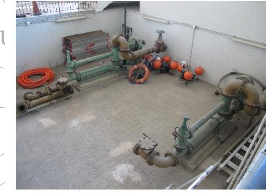
PHOTO 674: ABANDONED S.A.S PUMPS AT BELOW GROUND LEVEL (DATE TAKEN: 22 JULY 2016)
