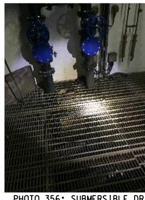
PHOTO 356: SUBMERSIBLE DRAINAGE PUMPS LOCATED IN THE BASEMENT OF WATER HEATER HOUSE (DATE TAKEN: 22 MAY 2017)
