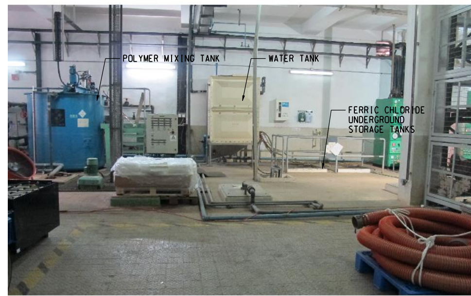
PHOTO 487: POLYMER MIXING TANKS AND FERRIC CHLORIDE STORAGE TANKS IN SLUDGE DEWATERING HOUSE (DATE TAKEN: 8 MARCH 2017)
