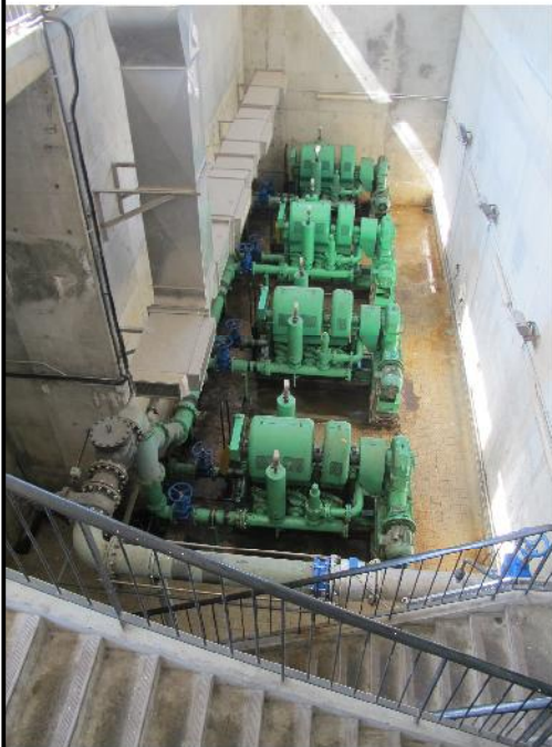
PHOTO 673: THICKENED SLUDGE PUMPS AT BELOW GROUND LEVEL (DATE TAKEN: 22 JULY 2016)
