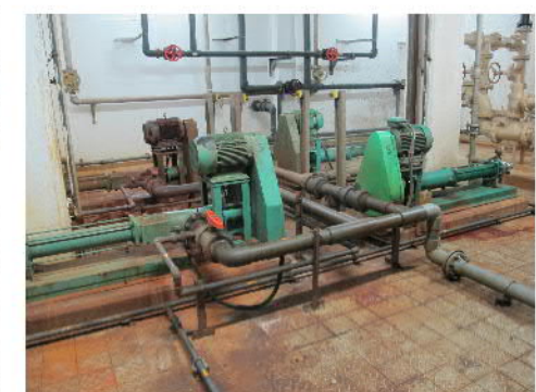
PHOTO 954: POLYMER DOSING PUMPS NO.1-4 IN THE BASEMENT OF SLUDGE DEWATERING HOUSE (DATE TAKEN: 22 MAY 2017)
