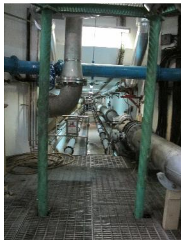
PHOTO 988: PIPE GALLERY IN THE BASEMENT BETWEEN WATER HEATER HOUSE AND METHANE COMPRESSOR HOUSE (DATE TAKEN: 22 MAY 2017)
