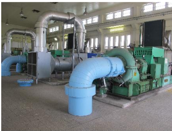
PHOTO 993: AIR BLOWERS ON THE GROUND FLOOR OF BLOWER HOUSE (DATE TAKEN: 22 MAY 2017)
