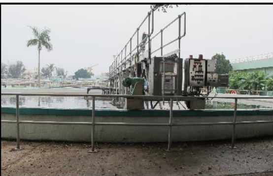
PHOTO 644: FINAL SETTLING TANK (DATE TAKEN: 8 MARCH 2017)
