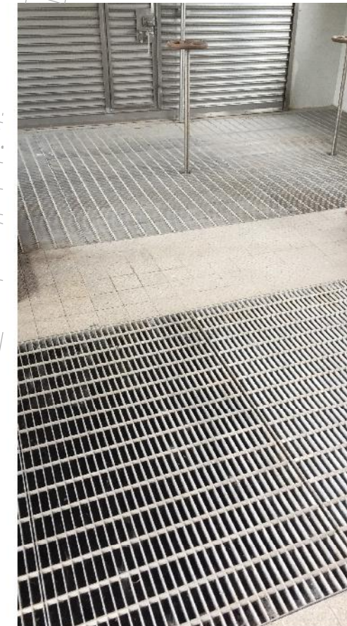
PHOTO 706: SUBMERSIBLE DRAINAGE PUMPS LOCATED UNDERNEATH THE ALUMINIUM OPEN MESH FLOORING AT BELOW GROUND LEVEL OF AUXILIARY PUMPING STATION (DATE TAKEN: 8 MARCH 2017)
