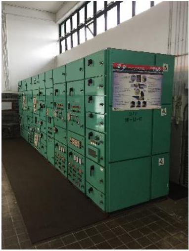
PHOTO 663: CONTROL PANEL IN CENTRAL CONTROL ROOM (DATE TAKEN: 8 MARCH 2017)
