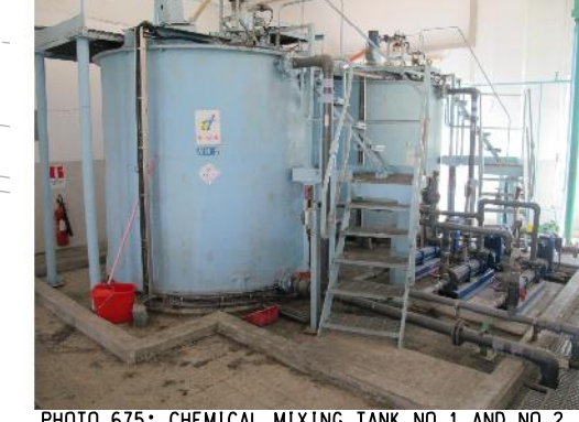
PHOTO 675: CHEMICAL MIXING TANK NO.1 AND NO.2 ON THE GROUND FLOOR OF SAS THICKENER HOUSE (DATE TAKEN: 22 JULY 2016)
