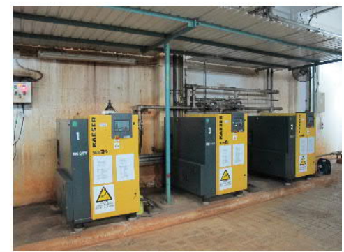
PHOTO 964: AIR COMPRESSORS IN THE BASEMENT OF SLUDGE DEWATERING HOUSE (DATE TAKEN: 22 MAY 2017)
