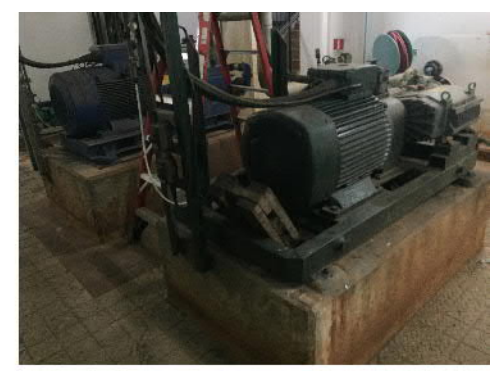
PHOTO 345: SLUDGE PUMPS NO.2-3 IN THE BASEMENT OF SLUDGE DEWATERING HOUSE (DATE TAKEN: 22 MAY 2017)
