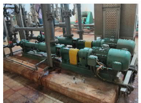
PHOTO 957: SLUDGE PUMPS NO. 4-5 IN BASEMENT OF SLUDGE DEWATERING HOUSE (DATE TAKEN: 22 MAY 2017)
