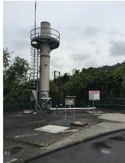
PHOTO 702: WASTE GAS BURNER (DATE TAKEN: 8 MARCH 2017)
