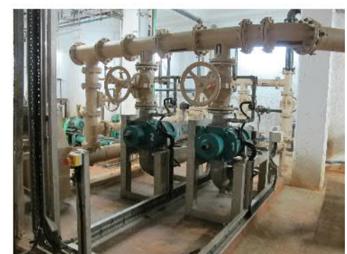
PHOTO 961: POLYMER DOSING PUMPS NO.5-6 IN THE BASEMENT OF SLUDGE DEWATERING HOUSE (DATE TAKEN: 22 MAY 2017)
